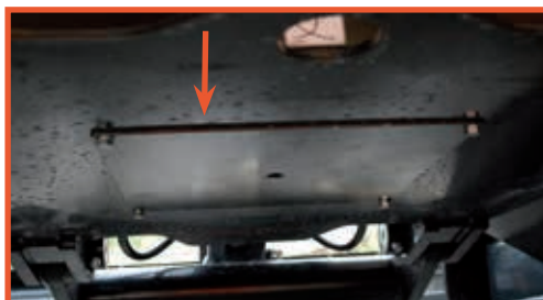
Protective panels over swivel joint.
