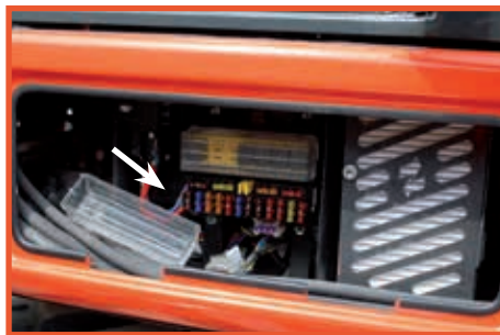
Fuses in a waterproof compartment and connection for external computer diagnostics.
